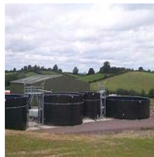
BELOW: A view of the New Duck Slurry Treatment facility at Silver Hill Foods.
